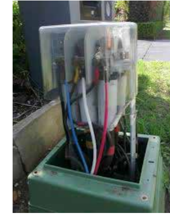
Additional Electrical Points For Events
