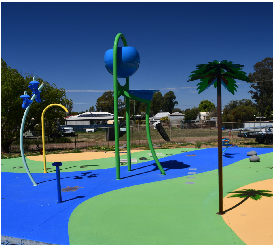
MAKING PROGRESS: The St George Splash Park is expected to be completed in time for the Christmas school holidays.
