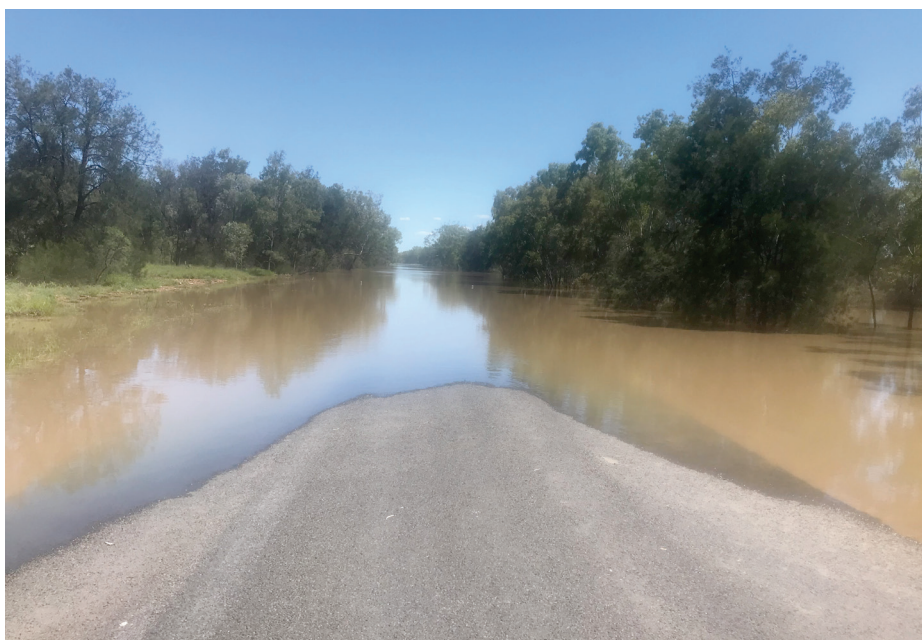
The Mungindi-Talwood Road also went under.
